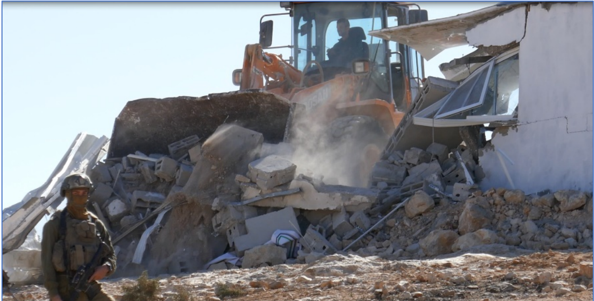
Isfey School demolished by Israeli bulldozer. (Photo Credit: EAPPI)
