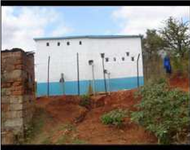
Kiko Kyaluma pumping station. Water is pumped from a subsurface dam and distributed to a distance of 18 Km with 10 water kiosks where the communities draw water.
